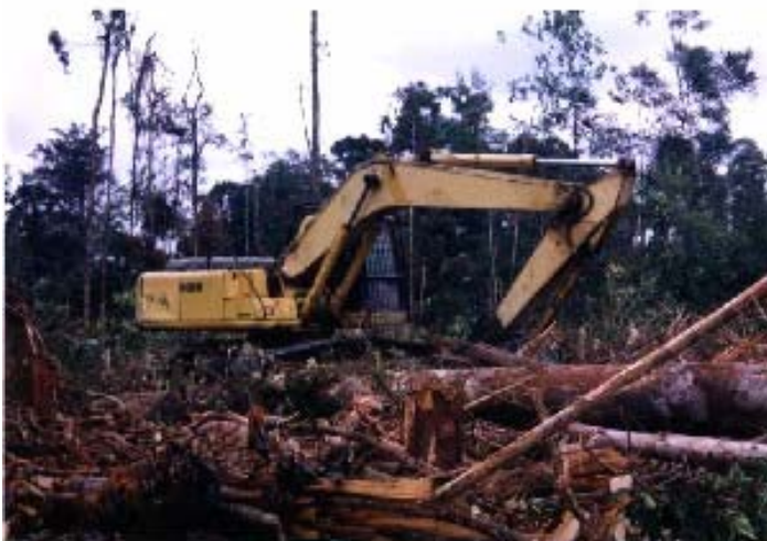
Figure 7. Excavator used in the professionally executed operations of Group 'W' (Photo taken on 1 June 2003)
